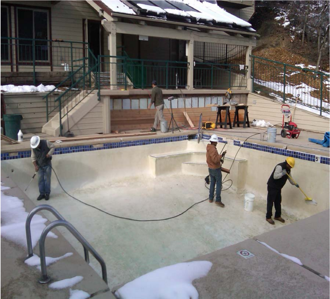
Power Washing the Pool and Replacing the Siding by the Pool Area
