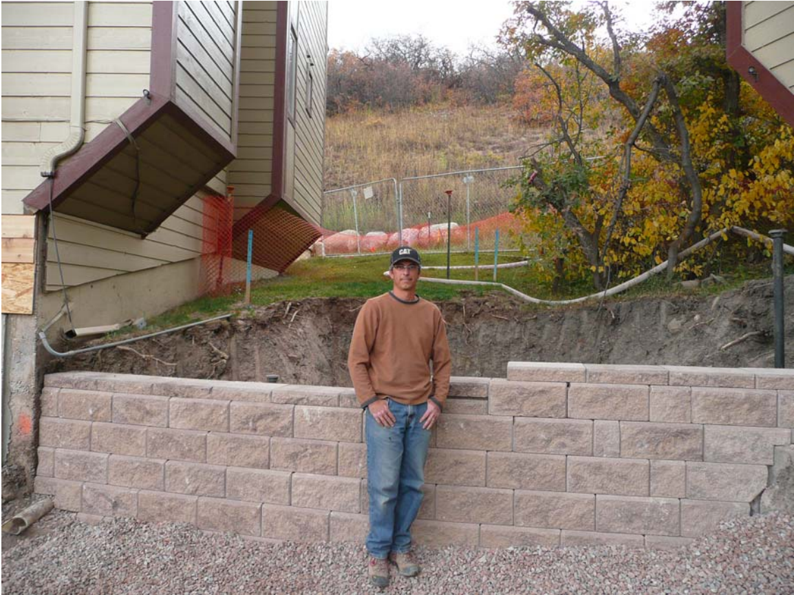
Bill Perry, Neenan Superintendent, in front of MSE wall between building C & D at bus turn around
