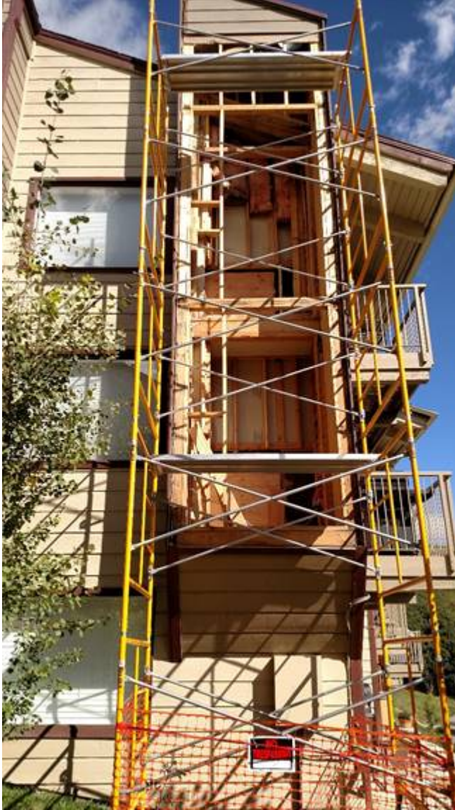
Figure 8 - Clean chase west side of Bldg J (except for good insulation)
