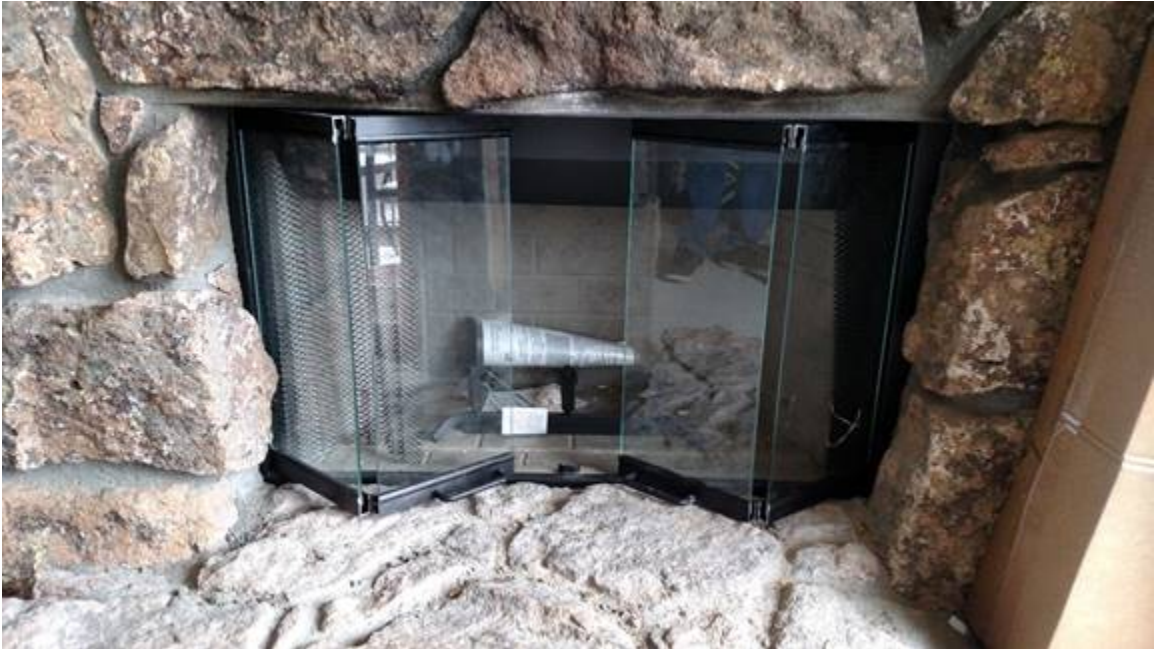
Figure 3 - this one still needs a little more work on the left side and bottom right (glass doors must open completely for correct install).
