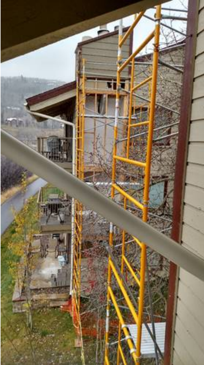
Figure 4 - Not the greatest picture but you can see the drywall work and flues
